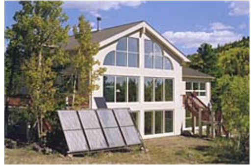
A home photovoltaic system provides power to the house and a solar domestic hot water system provides hot water for domestic and space heating use. Photo courtesy of the U.S. Department of Energy
